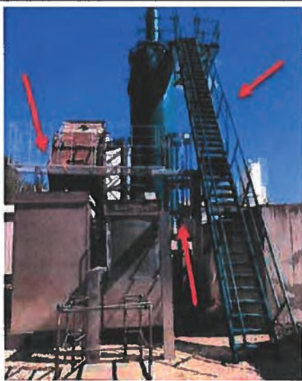
Stairways to stack platform
