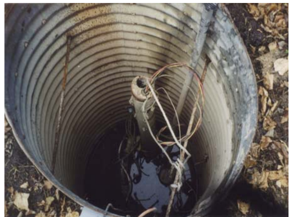
Well located in flooded well pit
