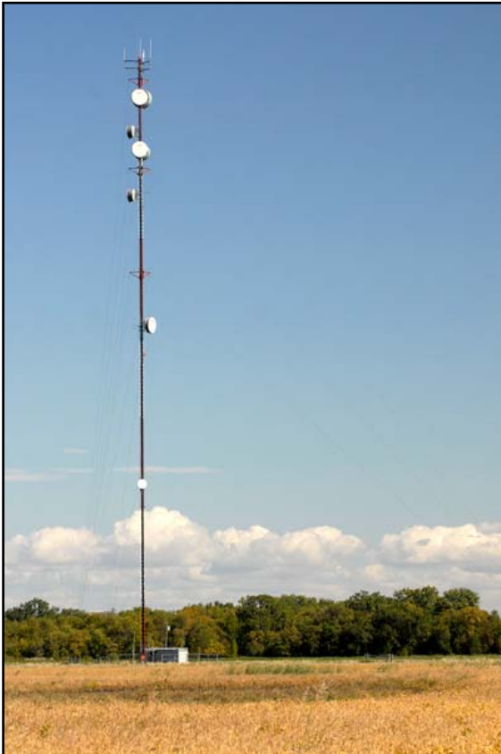
Image 3 - Cellular Communication Tower near High Bluff (height = 120 m)
