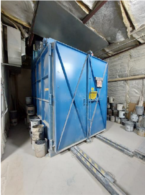
Photo 4: Guspro Inc. Oven with E Burners
