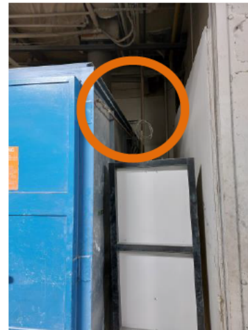
Photo 3: Disconnected Electrical Connection
