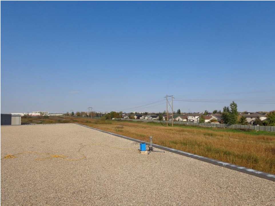
MP1 located at northeast corner of roof of Urbanmine building.
