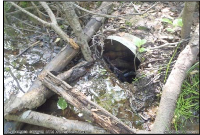
Figure 1: Stream crossing AD02, overgrown culvert.
