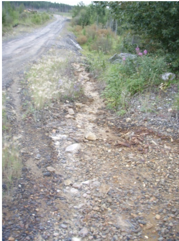
Figure F4: Runoff on Northeast side of Arsenopyrite Residue Stockpile
