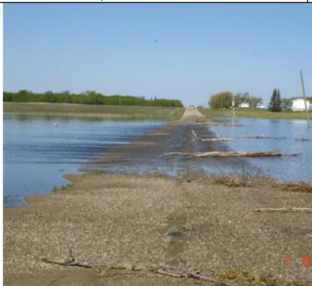
Figure 12 - Flooding and damage - Road 94N
