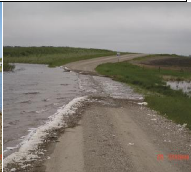
Figure 13 - Flooding and damage - South Lake 2011
