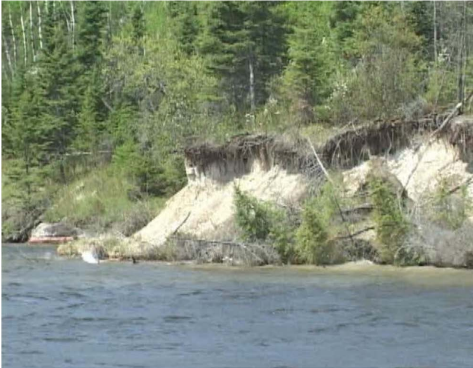
Photo 7.17: Active Clay Bank Failure
