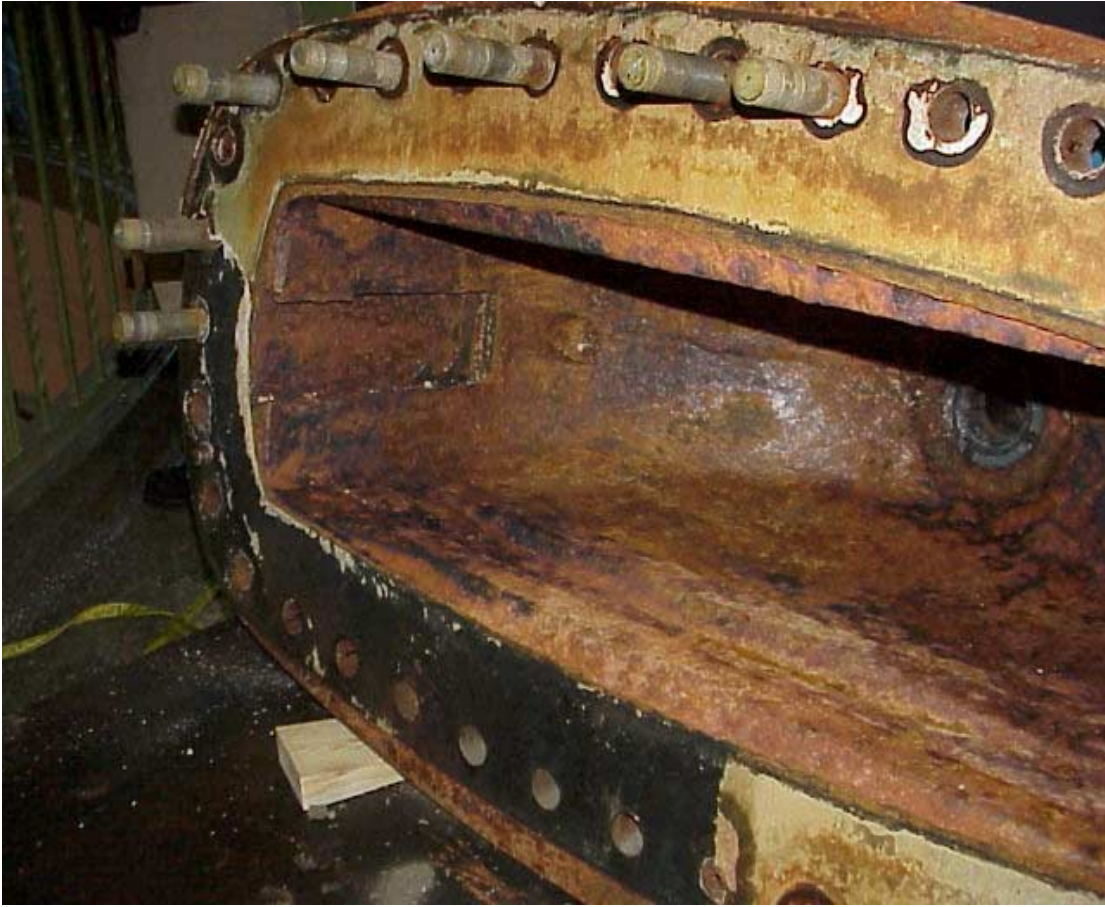
Photo 511 Top Bonnet of suction gate valve. Left side of interior of bonnet shows valve guide bar is missing.
