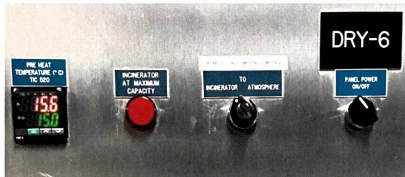
Fig.1: Dryer control panel
