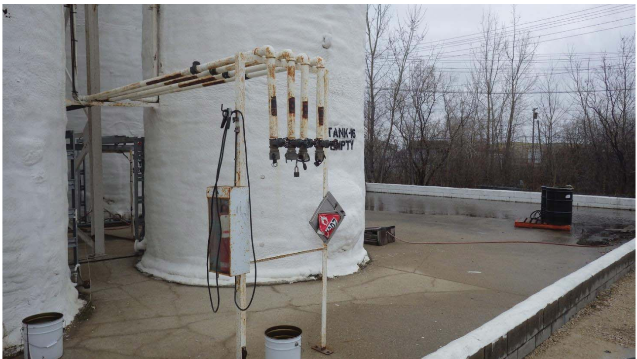
Photo 8. Northwest view of tank farm close-up showing filling hook-up, cement pad and cinder block containment dike.
