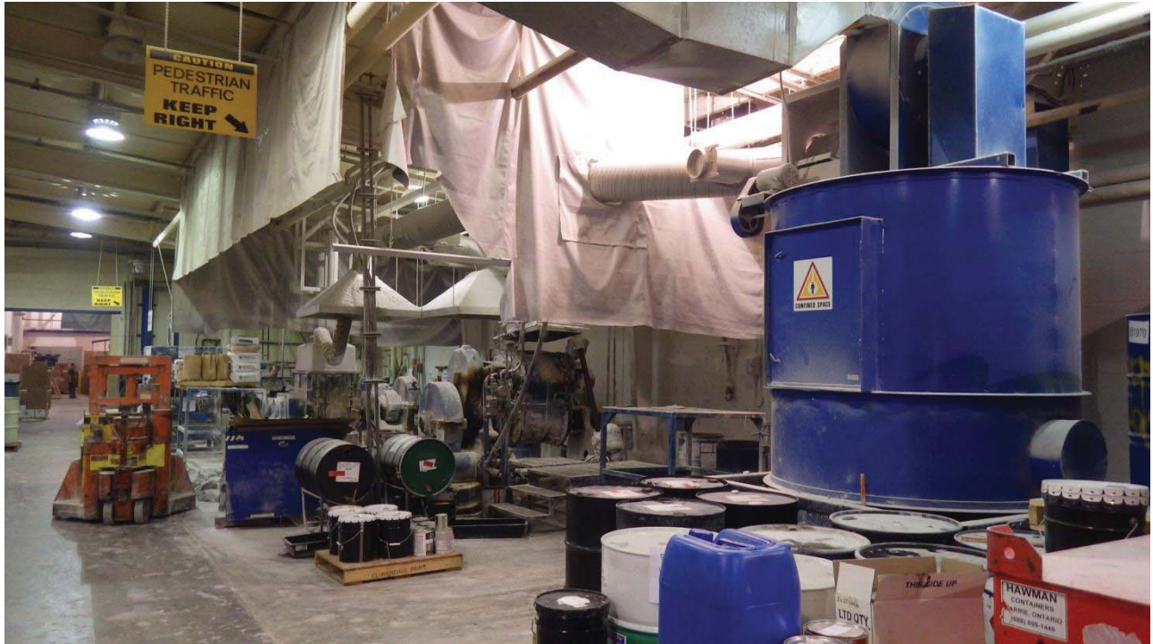
Photo 25. Sealant/caulking manufacturing area with baghouse in foreground.
