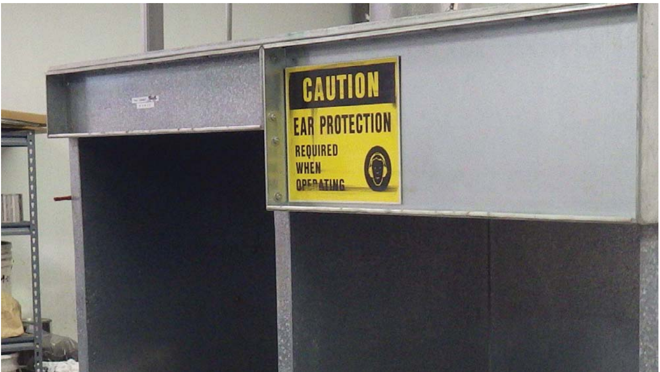
Photo 26. Signage warning about requirements for hearing protection.
