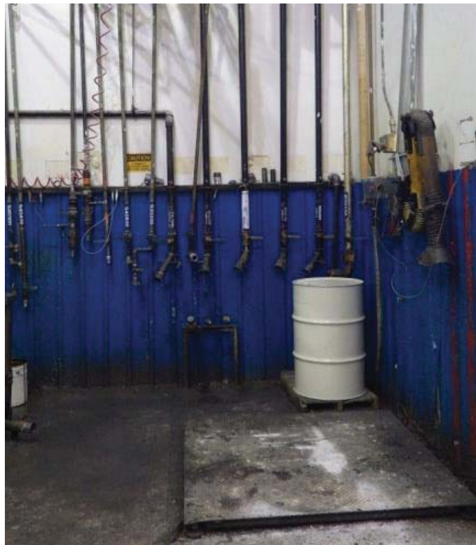
Photo 14: Piping inside of manufacturing facility for materials coming in from the tank farm.
