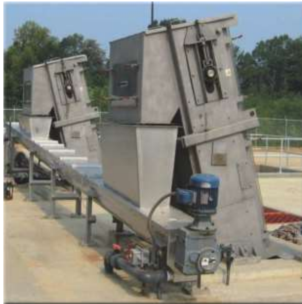
Figure 3.2: Mechanical Screens (Image from Headworks)
